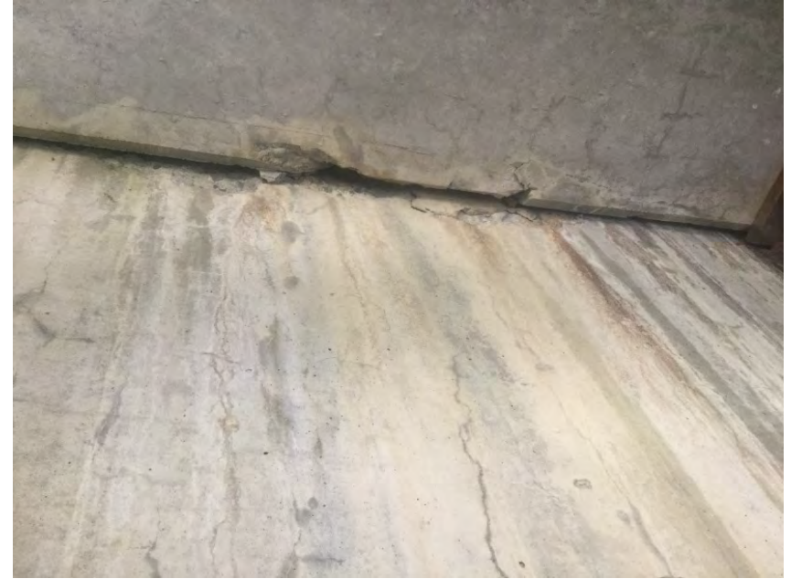
Minor spalling noted on left bank wall and panel 1
