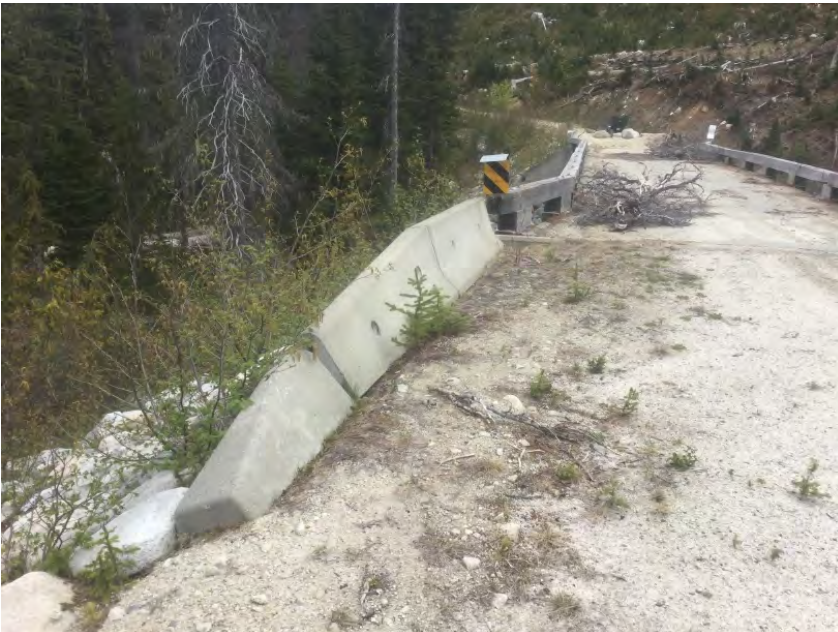
Downstream left approach barriers failing
