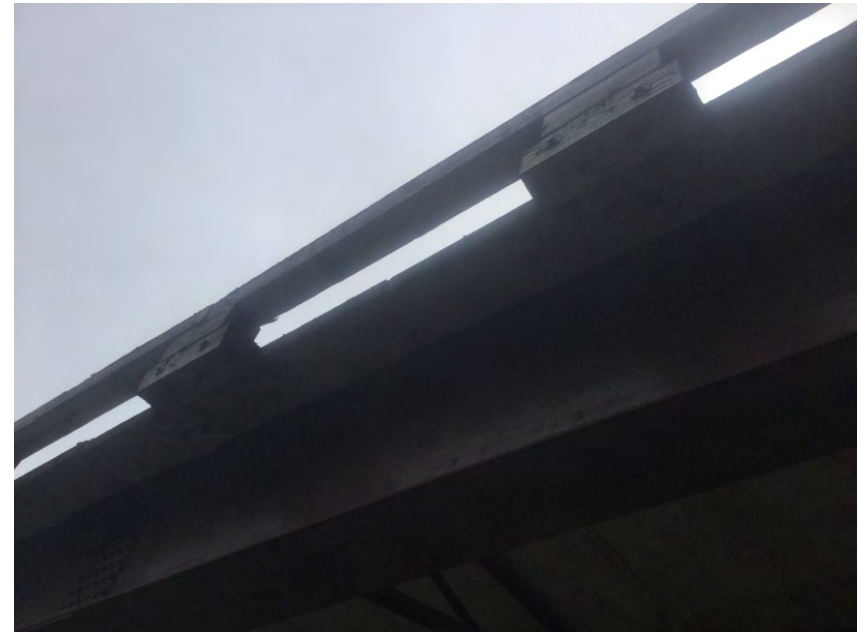
Damage noted under 2 panels with rebar showing
